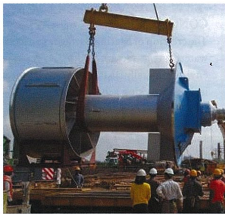
Drainage pump at Marina Barrage.
