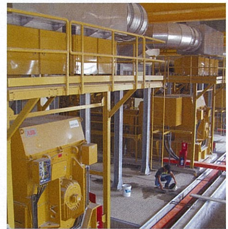
Diesel engine-generators in the electrical building.
